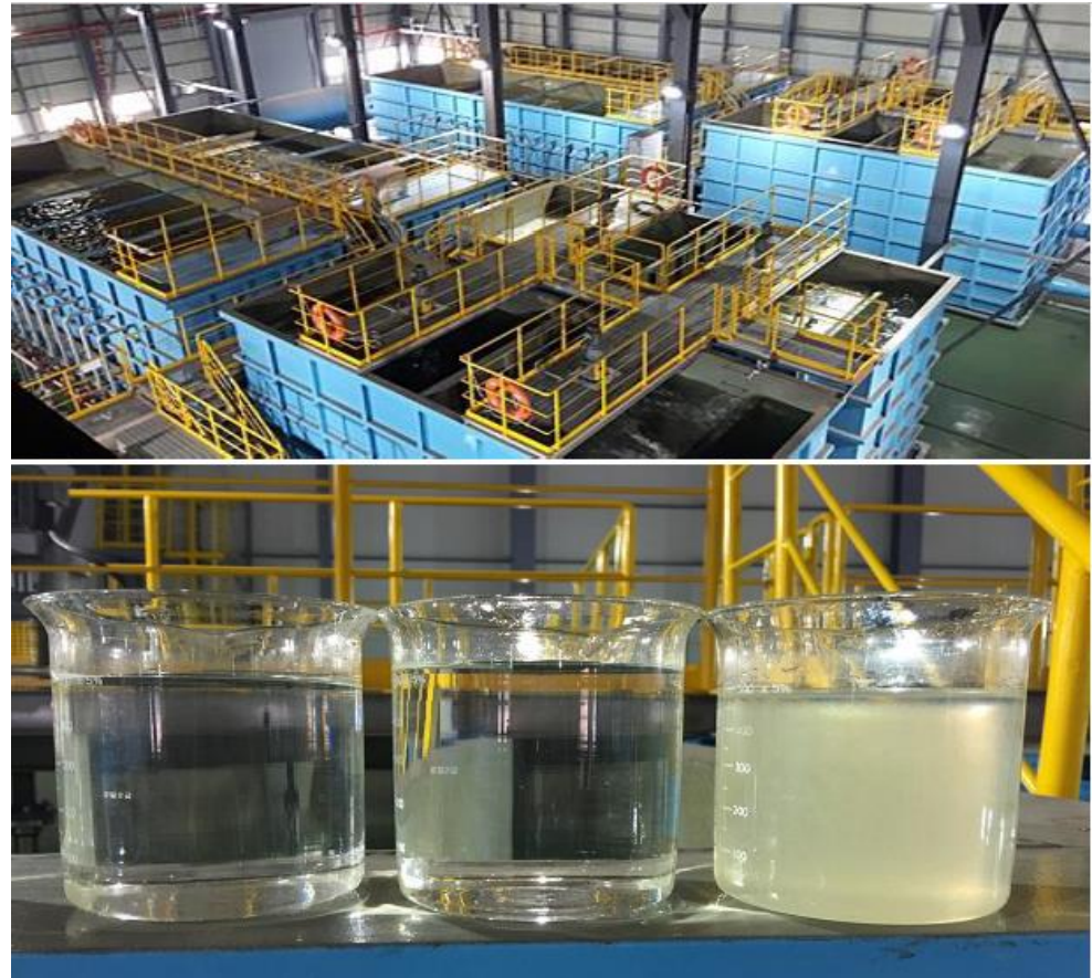
Figure 1 – Cloth filtration plant with chemical coagulation at Hyundai Steel (Dang-jin, South-Korea). Below from left to right: raw water, treated water and backwash water.
